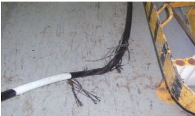
Figure.5 The recovered un-buried cable of damaged fibres
